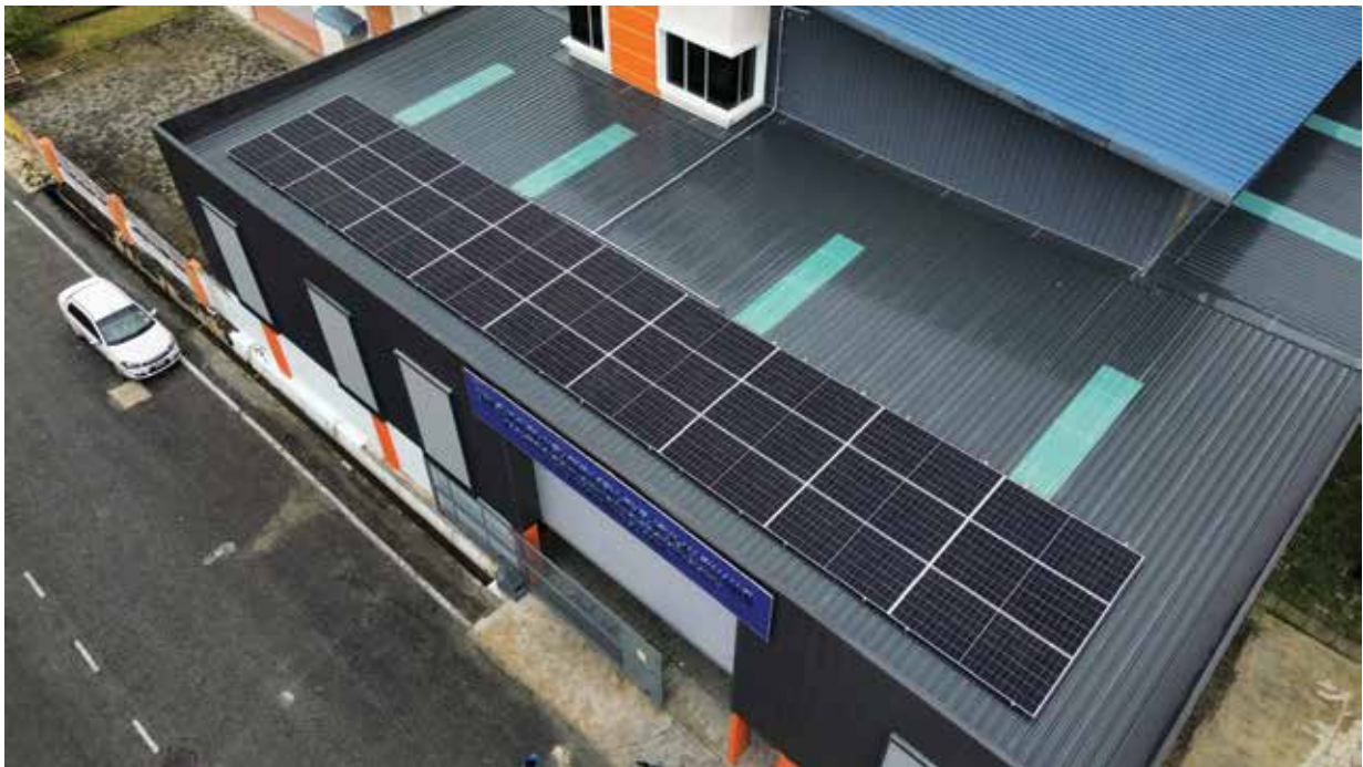
Solar Panel at Penang Branch
