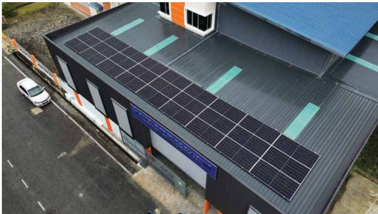
Solar Panel at Penang Branch
